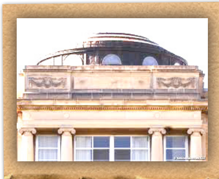
The Copperdome atop the Administration Building at Shorewood High School. The copper was refurbished in 2021.
