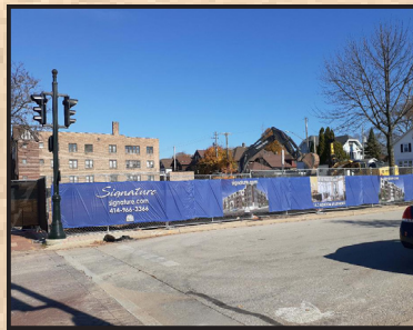
The apartment complex currently under construction at Oakland Ave. and Lake Bluff Blvd., site of the former North Shore Bank building.
